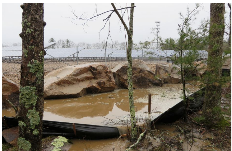
Example of runoff at a solar installation in Rhode Island caused by lack of temporary swales and sediment traps according to RI DEM.
